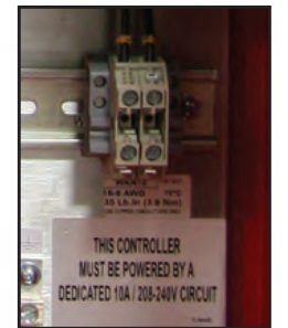
• Incoming power connection
